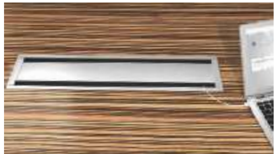
Open the wiring at both sides of the line box of conference table
